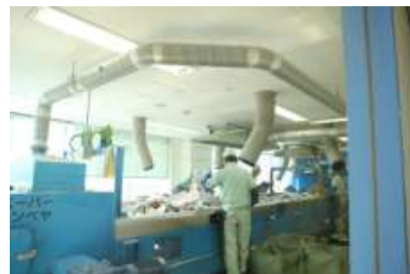
Figure 1: Kawasaki City recycling and treatment facilities
